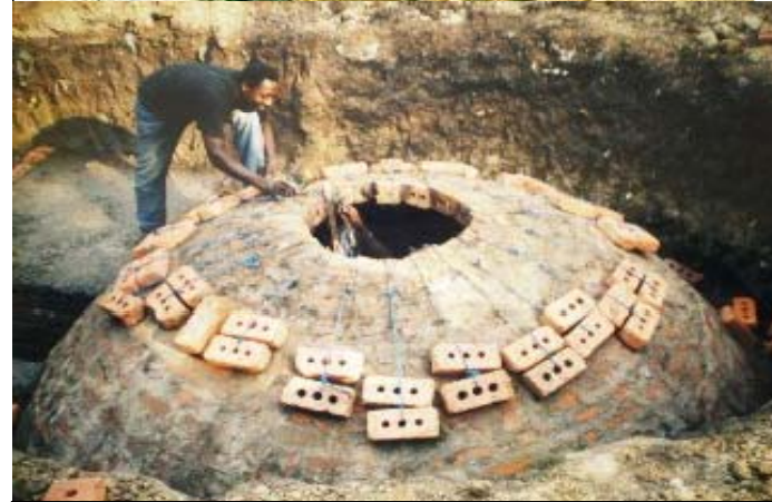
Above: Floating drum Biogas plant, Burkina Faso Below: Fixed Dome Plant under construction in Ghana. Photo: GTZ/REES
